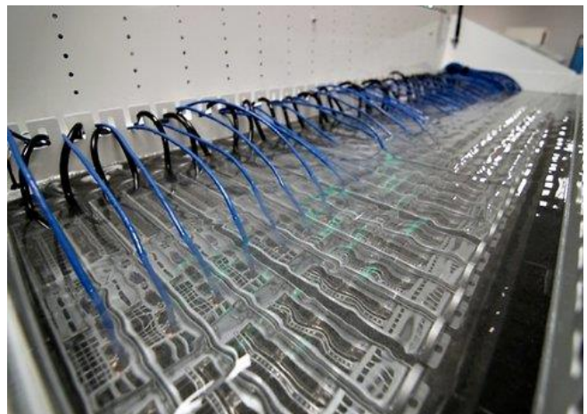
Submersion Cooling Bath
